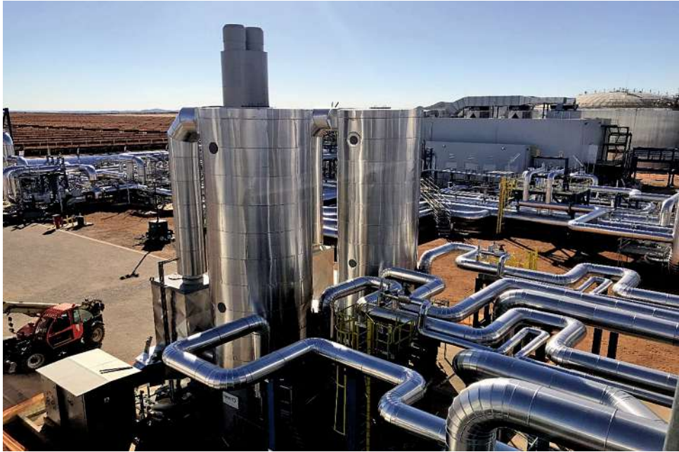
Fig. 6 Two bottom-fired thermal oil heaters (fired boilers) with a capacity of 7 MW each, combustion air pre-heater, stack for 100 MW CSP plant “Ilanga” nearby Upington in South Africa [Source: heat 11].
