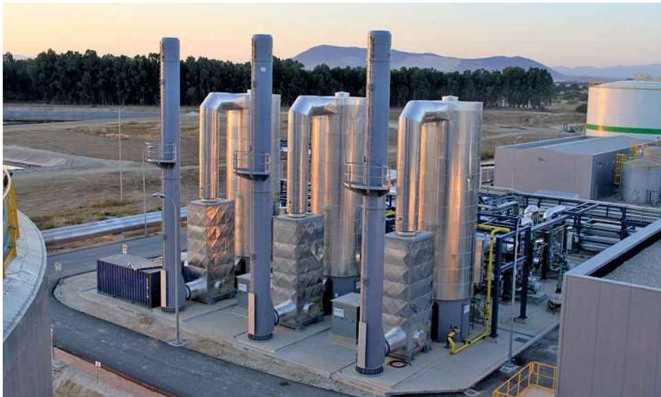
Fig. 5 Three bottom-fired thermal oil heaters (fired boilers) with a capacity of 17 MW each, combustion air pre-heater, stack for CSP plant “Los Arenales” nearby Seville in Spain [Source: heat 11].
